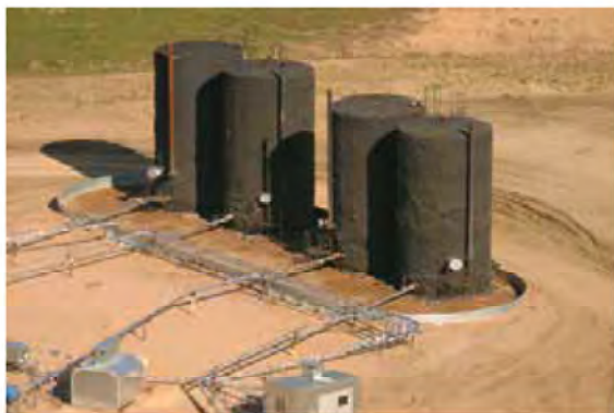
Figure 22. Secondary containment system in Alberta, Canada
