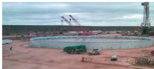
Figure 20. Enviro Liner® 6030 Frac Tank Liner, West Texas.
