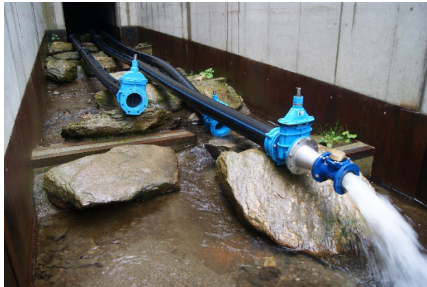
Figure 172-4 Controllable Outlet Pipes with Remotely Controlled Charges at the Valves (The proposed system for Cougar Creek will feature longer pipes to ensure that the charges are outside of the Structure footprint)
