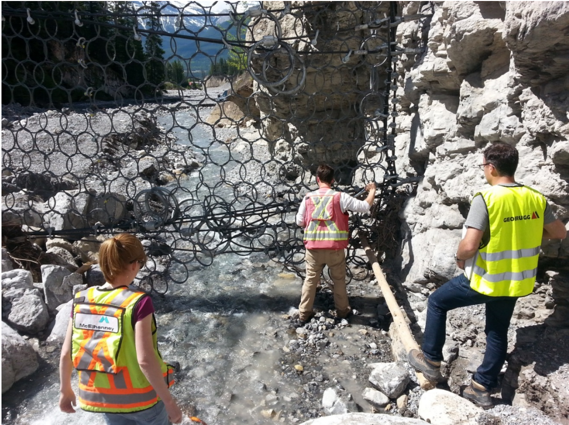
Figure 66-3 Downstream View of Modified Debris Net with low Flow Opening (Town of Canmore photograph, May 2014)
