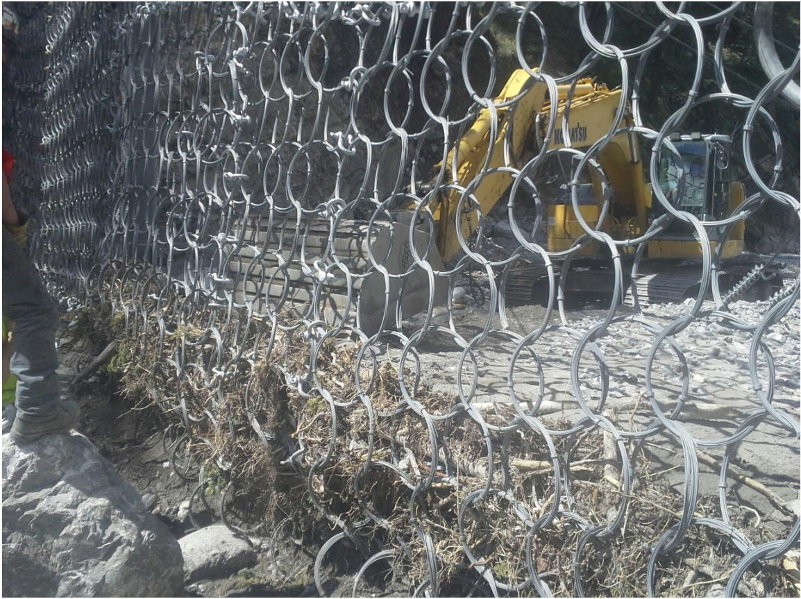
Figure 66-2 Debris Accumulation Upstream of the Debris Net (Town of Canmore photograph, May 2014)
