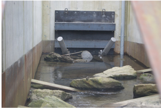
Figure 172-1 Temporary Shut-off Plate, Placed at the Intake Throttle, with Inflow Strainer Feeding the Downstream Pipes going through the Bottom Outlet Structure
