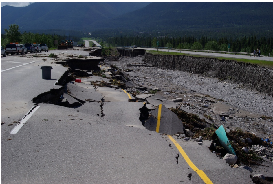
Photo A-31. Damage to Highway 1 as a result of the 2013 debris flood. View is looking east. Photograph courtesy of the Town of Canmore.
