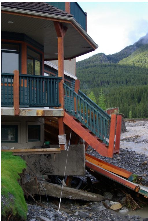
Photo A-10. Structural damage sustained to home along Eagle Landing. Photograph courtesy of the Town of Canmore.
