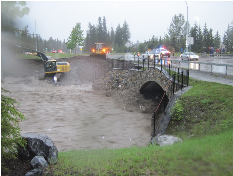
Photo A-2. On right bank of Cougar Creek looking to left bank at the Elk Run Boulevard culvert. Emergency efforts to protect the outflanking of the culvert are underway. Photograph courtesy of the Town of Canmore.
