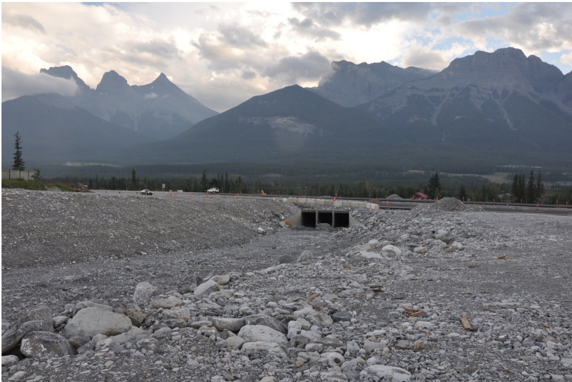
Photo 2-2. Downstream view of the culvert inlet at Highway 1. BGC photograph of July 23, 2013.
