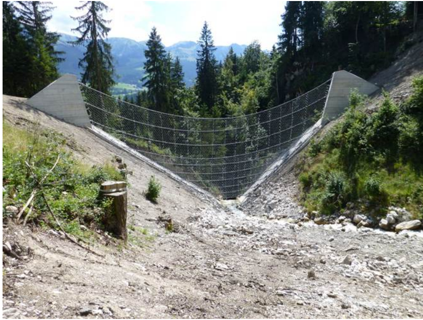
Photo 8-1. Downstream view of 14 m high debris flow net. Photograph courtesy of Geobruigg North America, LLC.
