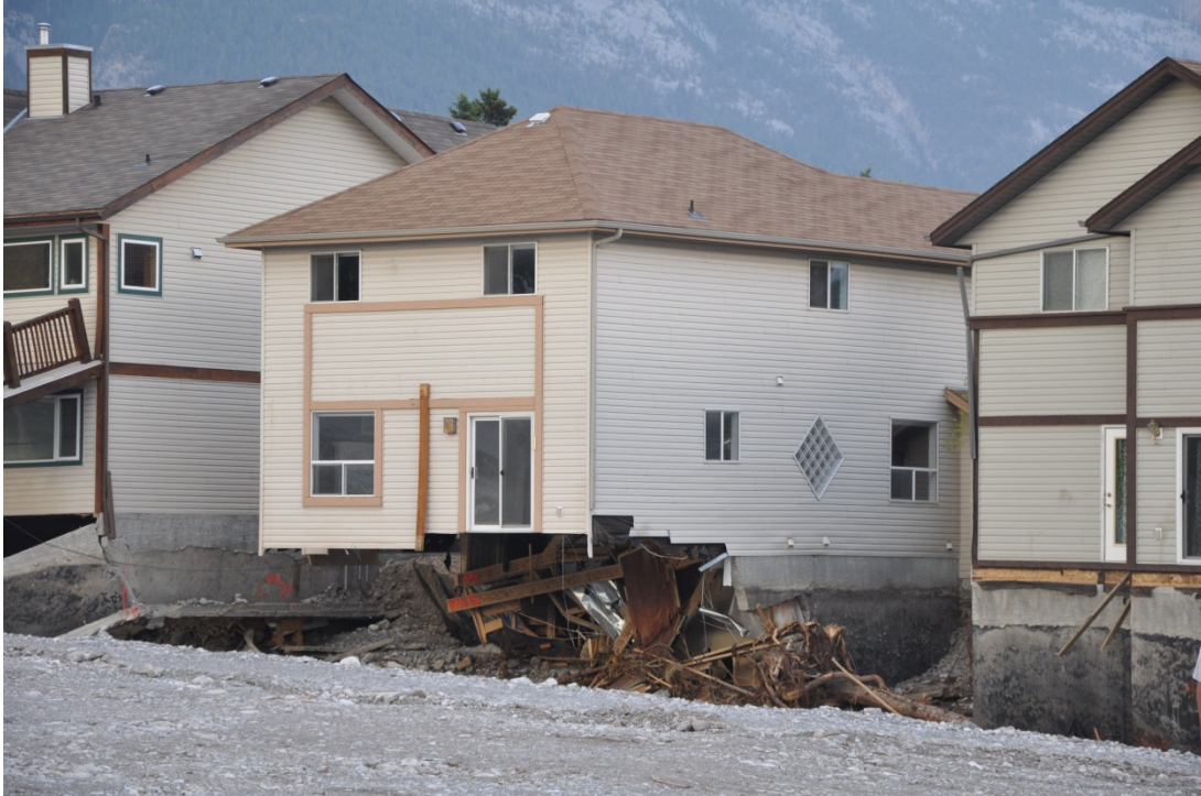
Photo A-19. Damage sustained to home along the left (east) bank of Cougar Creek along Grotto Road. BGC photograph of July 23, 2013.
