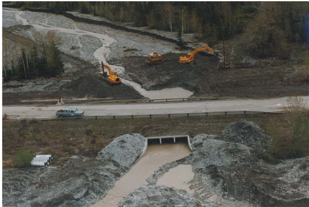
Photo 3-8. Excavation activities at Highway 1A following the dam failure. Photo courtesy of Kent Berg, Alberta Environment and Sustainable Resource Development. May 26, 1990.
