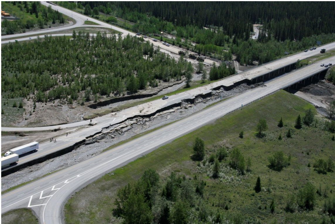
Photo A-30. Aerial view (looking northeast) of Highway 1 following the 2013 debris flood. Photograph courtesy of the Town of Canmore.
