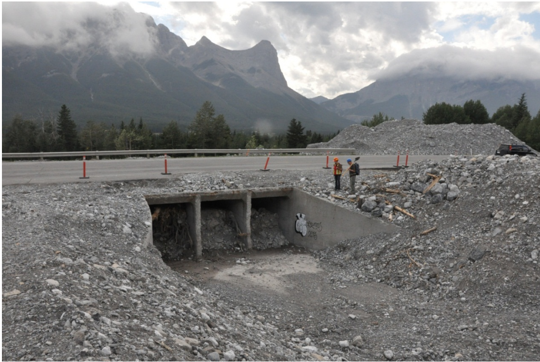
Photo 2-3. Culvert inlet at Highway 1A. The culvert was full of debris at the time of the site visit. BGC photograph of August 8, 2013.
