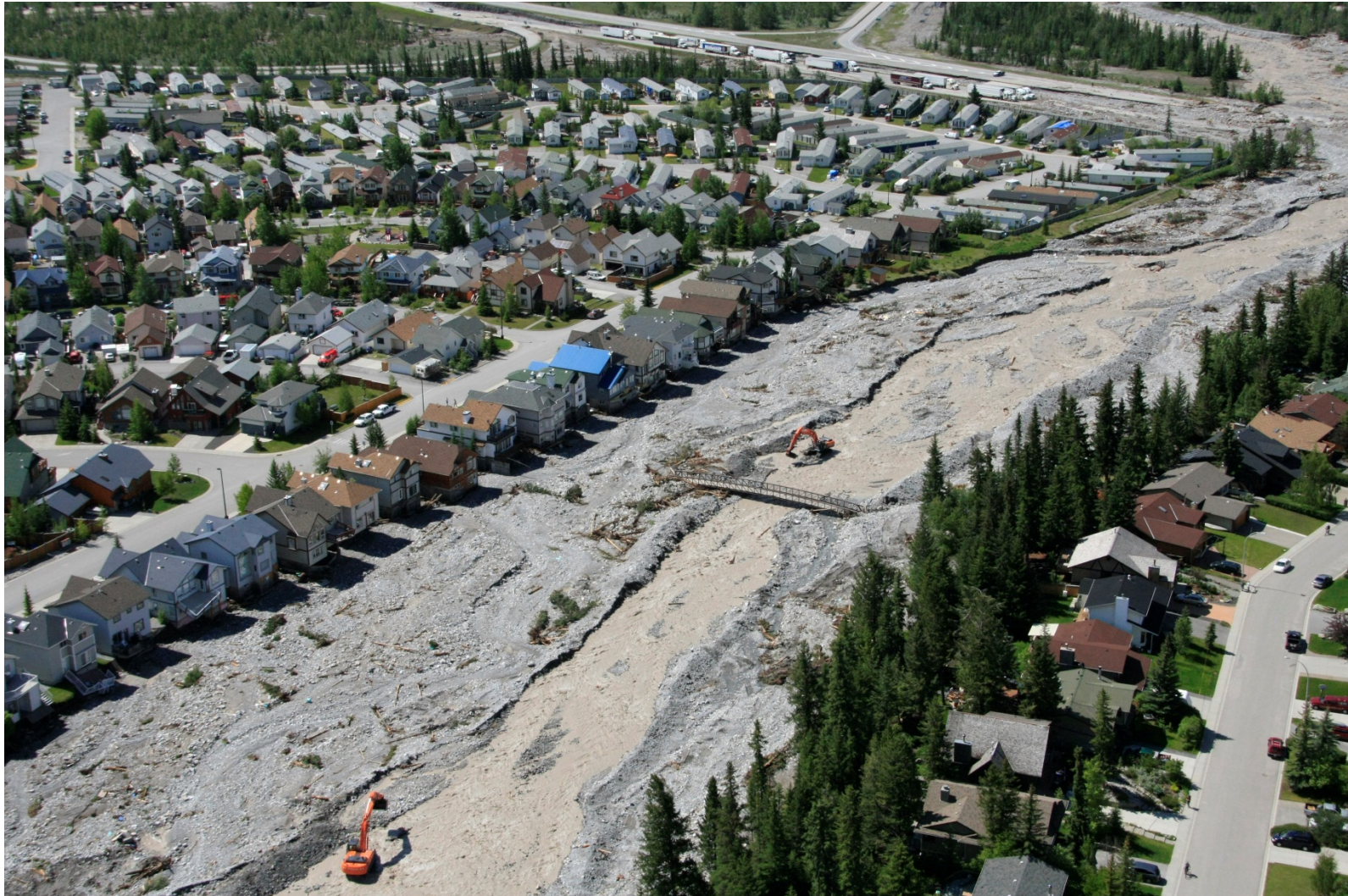
Photo A-27. Aerial view of restoration efforts along Cougar Creek between Elk Run Boulevard and Highway 1 following the 2013 debris flood. Photograph courtesy of the Town of Canmore.
