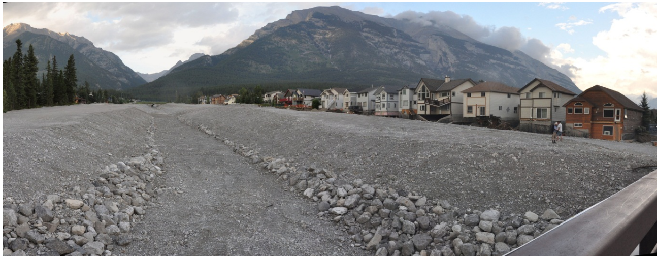
Photo A-36. Upstream view of reconstructed Cougar Creek channel from the pedestrian bridge. BGC photograph of July 23, 2013.
