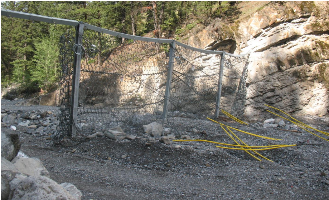
Figure 2: Debris-Net at the intended location of the debris-flood retention structure as part of short-term mitigation measures (CHT 2015)
