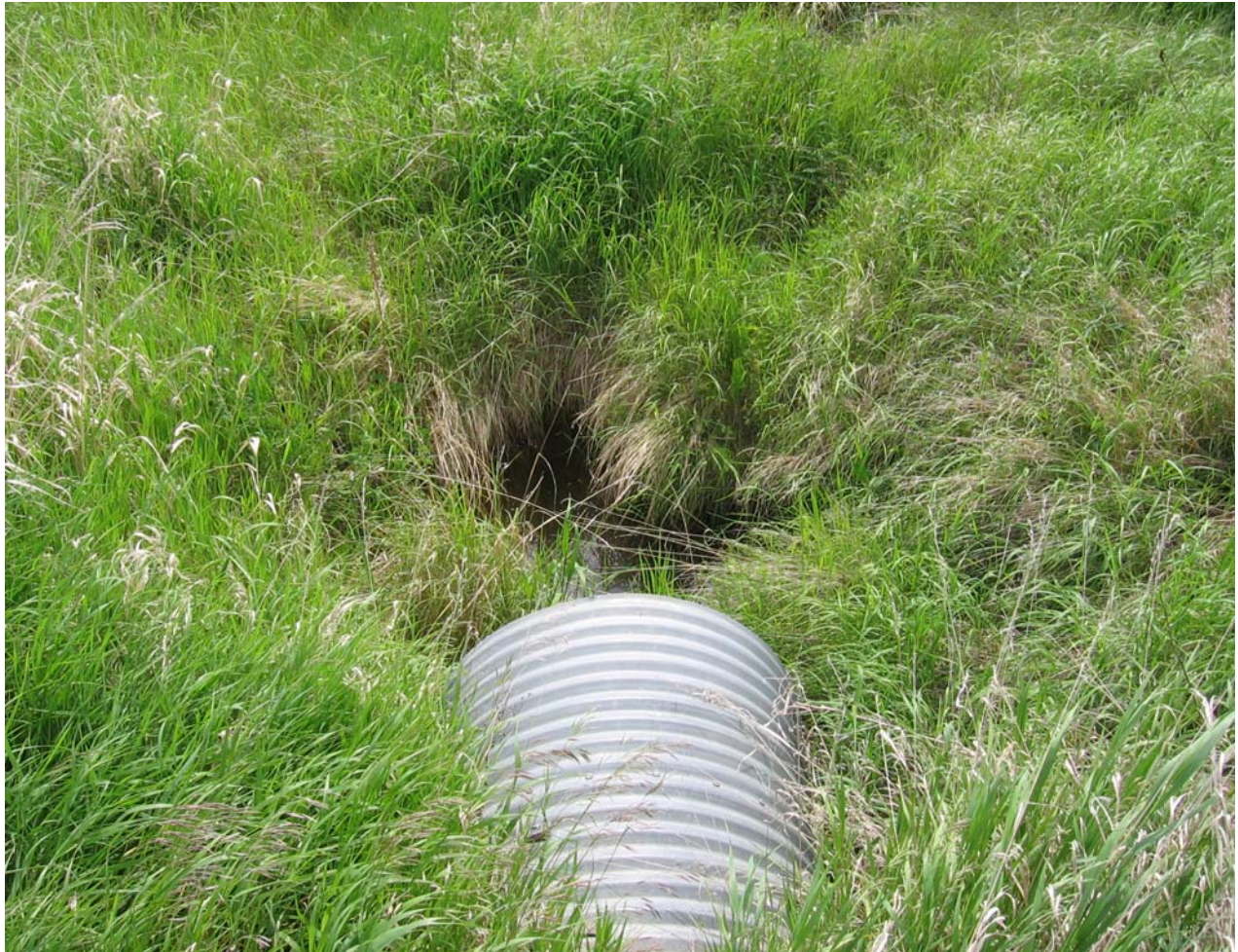
Photo III-7: Surface Water Quality Monitoring Location SW7 looking North (June 14, 2006). Conveyance under the CN Railway is via a 914 mm Corrugated Steel Culvert
