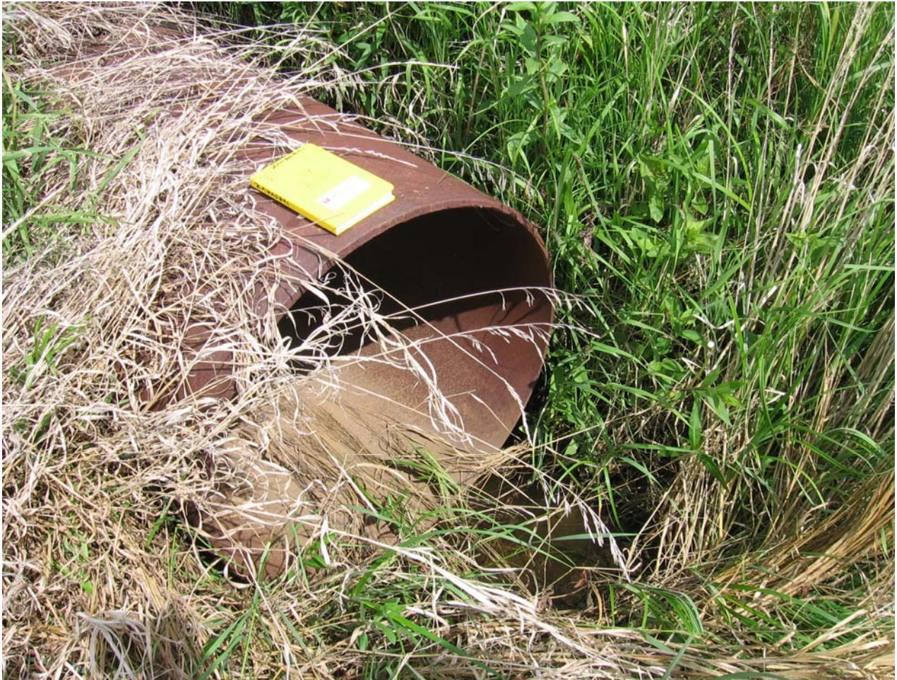
Photo III-6: Surface Water Quality Monitoring Location SW6 looking North (June 14, 2006). Conveyance under the CN Railway is via a 762 mm Steel Pipe
