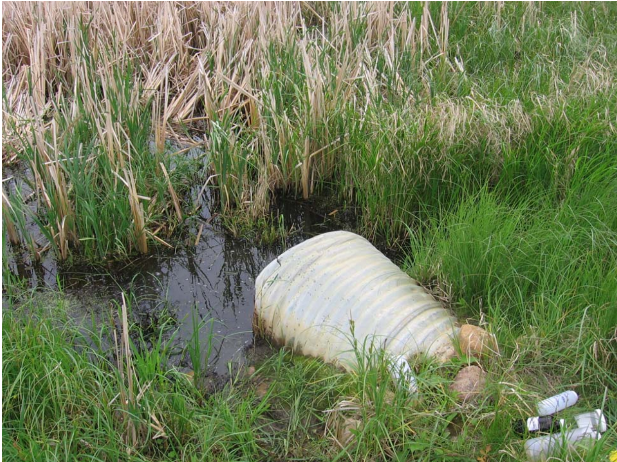
Photo III-1: Surface Water Monitoring Location SW1 Looking East (June 14, 2006). Conveyance under R.R. 202 is via a 609 mm Corrugated Steel Culvert
