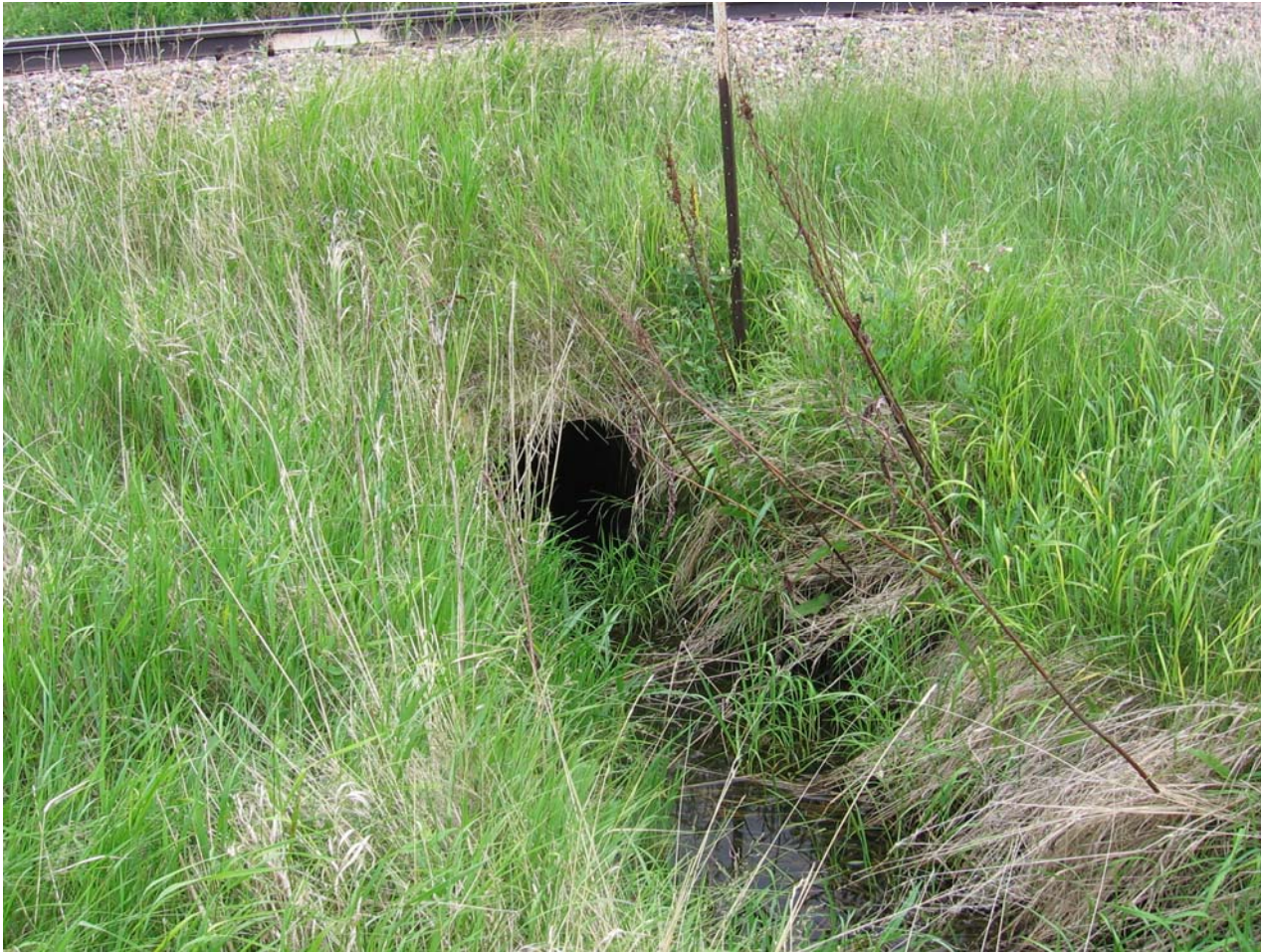
Photo III-4: Surface water monitoring location SW4 looking south (June 14, 2006). Conveyance under the CPR Railway is via a 304 mm Corrugated Steel Culvert (shown) and a 610 mm Corrugated Steel Culvert (immediate left of photo)
