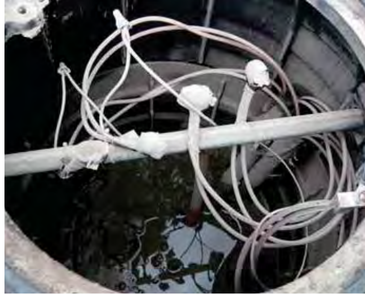
Fig. 12 - In-Grade JB - debris buildup
