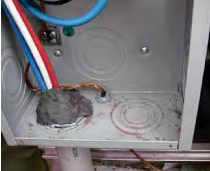
Fig. 3 - Main Breaker enclosure - Dry
