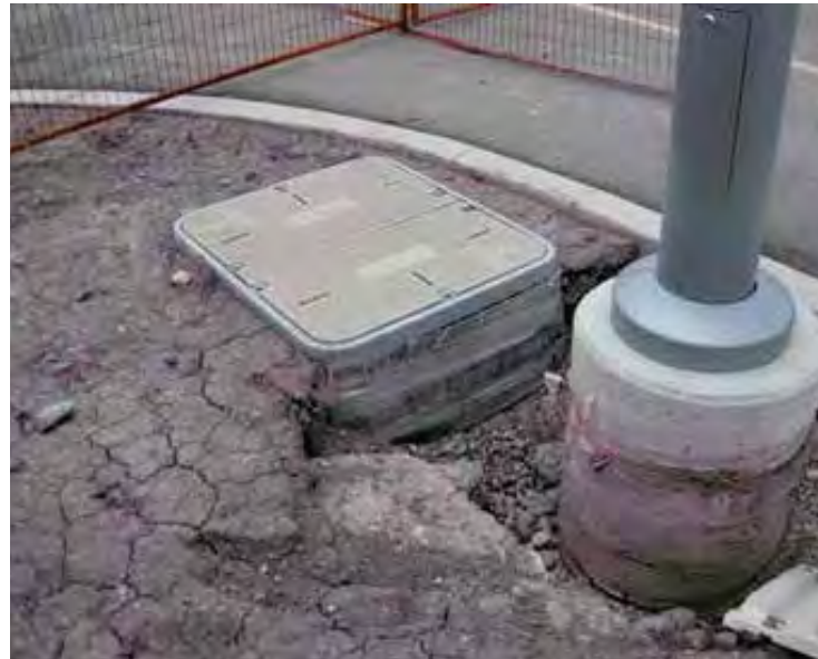
Fig. 14 - ITS Pull box erosion
