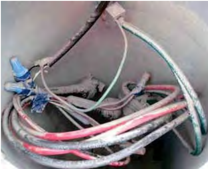
Fig. 5 - Hess Night Element Hand Hole - Submerged
