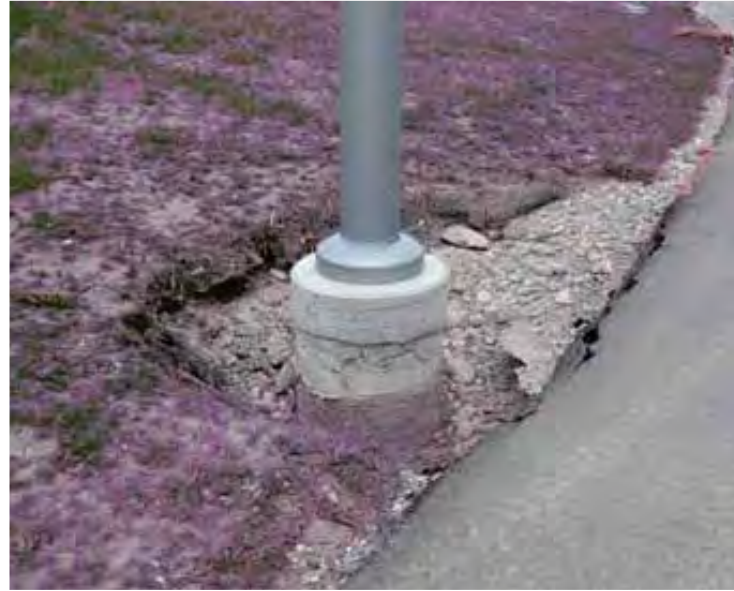
Fig. 4 - Hess Night Element Base Erosion
