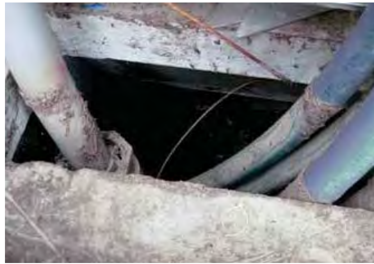
Fig.2 - Main panel incoming conduits – Water level indicated by debris buildup
