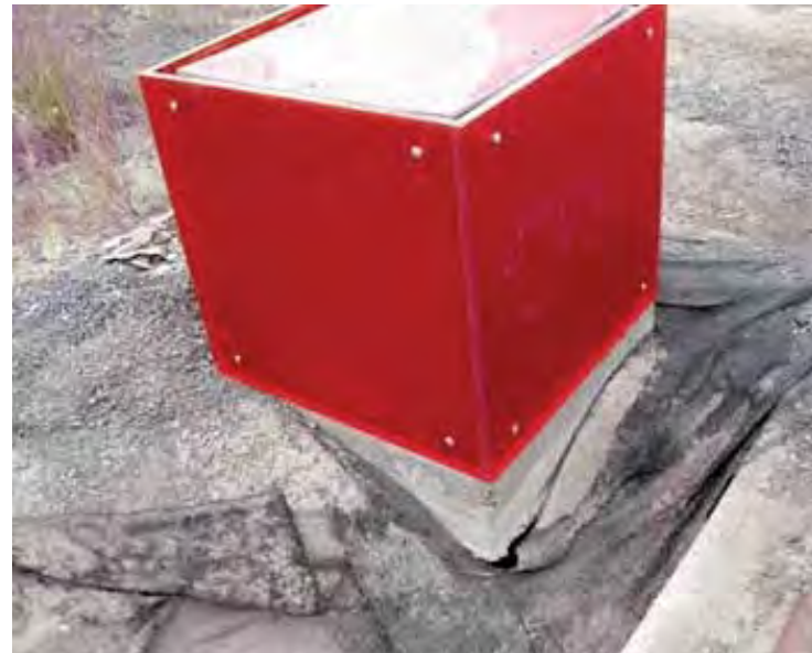
Fig. 10 - Cube Foundation Erosion
