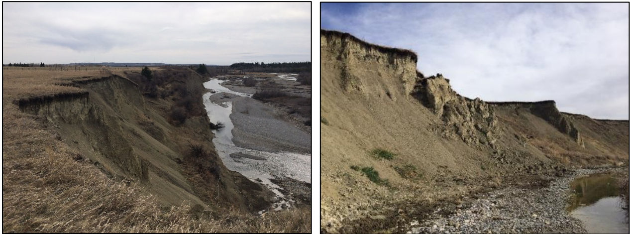
Figure 19. Slope Instability observed in glacial units on the Elbow River Valley downstream of the dam
