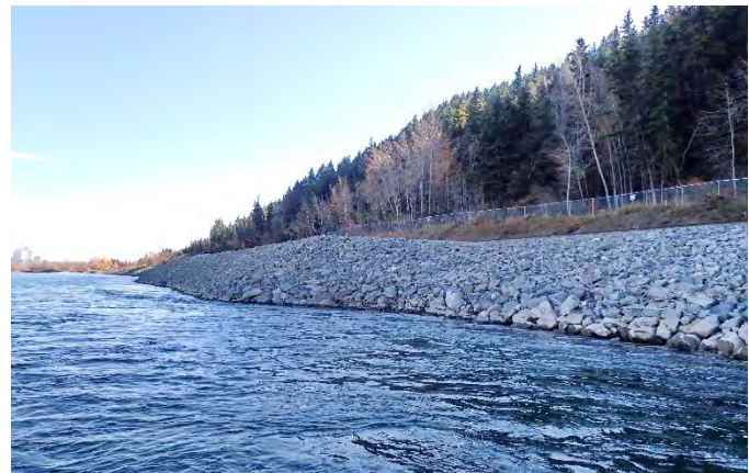
Riprap bank protection along the Bow River
