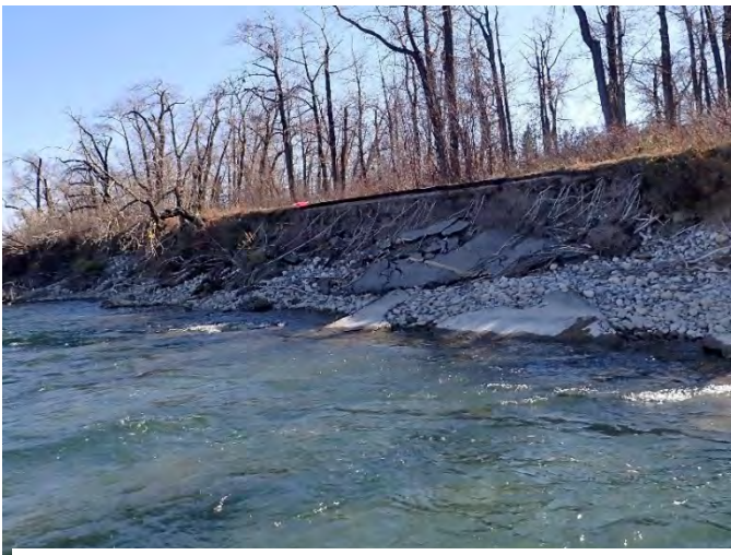
Bank erosion on the Bow River
