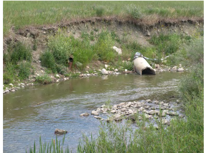
Bank erosion along Nose Creek
