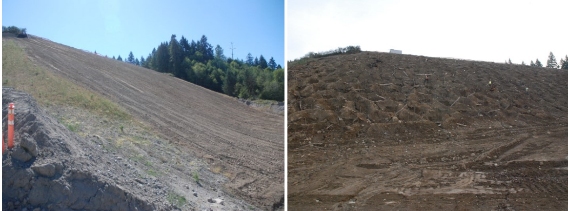
The hill was re-sloped (left) and then made rough and loose (right) with an excavator (photos courtesy David Polster).
