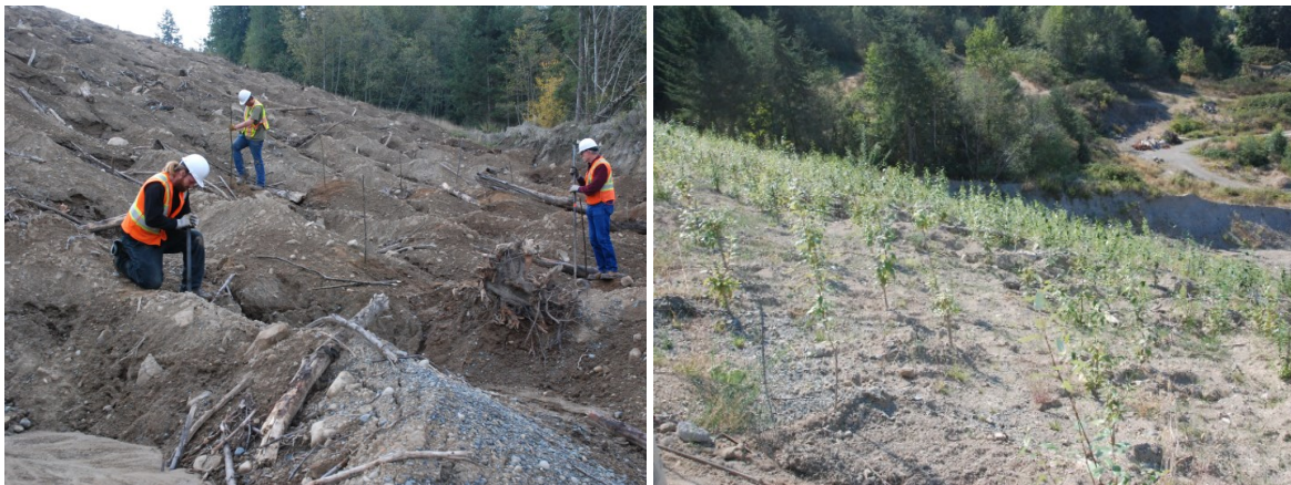
2500 live poplar stakes were planted in November 2014 (left). The stakes had good survival the following year and the slope remained stable (right) (photos courtesy David Polster).
