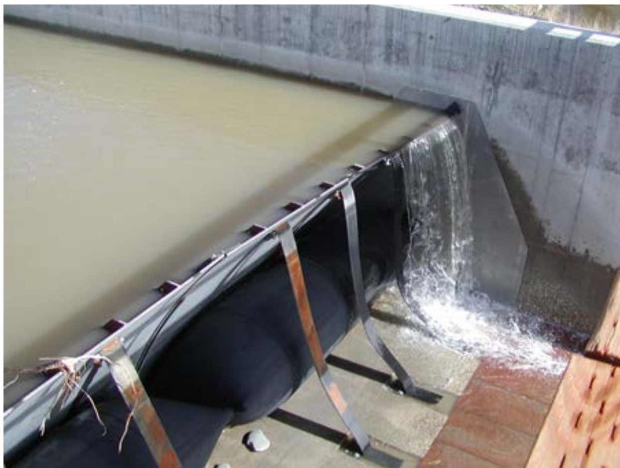
Figure 3-4 An Obermeyer Crest Gate in Raised Position
