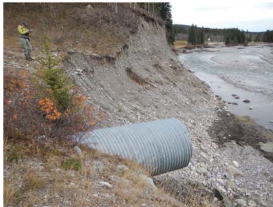
Plate 1: 5 m perched culvert at confluence with Elbow River presenting a fish migration barrier. 21 October 2014
