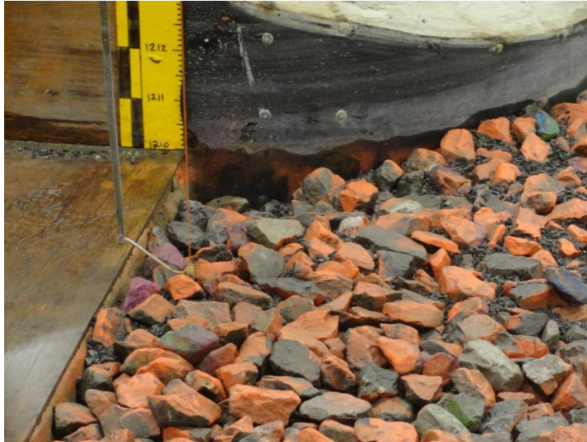
Figure 117. Scouring of the 440kg rip-rap at RHS of the service spillway inlet.
