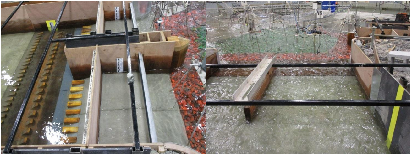
Figure 156. Diversion inlet structure (left) and service spillway (right) during the 160 m 3 /s flow condition.
