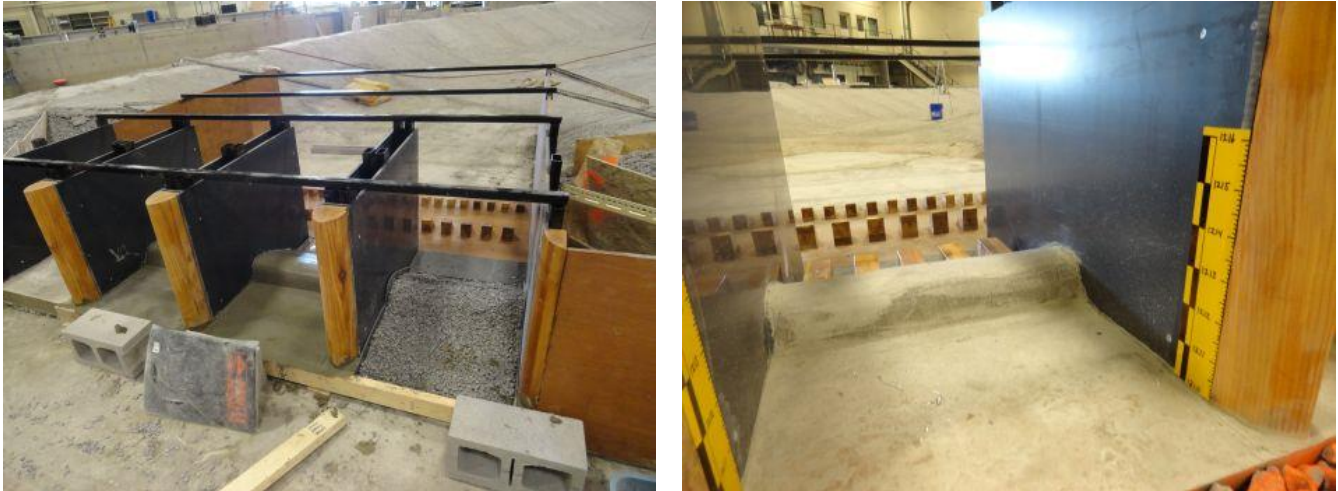
Figure 40. Left: forming the concrete apron. Right: concrete apron and front chute blocks installed.
