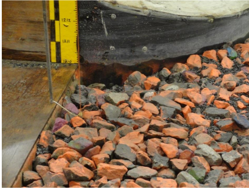
Figure 117. Scouring of the 440kg rip-rap at RHS of the service spillway inlet.
