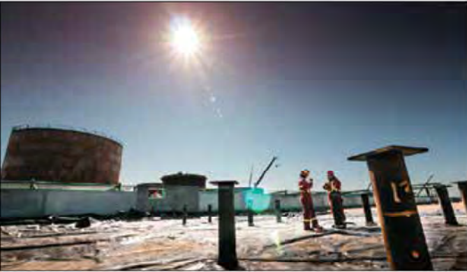
Figure 16. Double Lined secondary containment system lined with Enviro Liner® 6030
