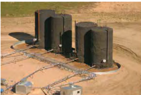
Figure 22. Secondary containment system in Alberta, Canada
